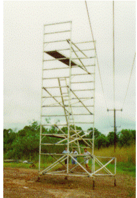
Photo used from archives showing scaffolding in contact with overhead powerlines
