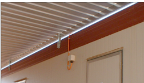
Caption: Junction box for a mains connection on a relocatable dwelling
