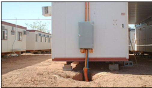
Caption: View of external switchboard on relocatable dwelling
